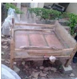
Fig.1. Constructed Wetland Unit
